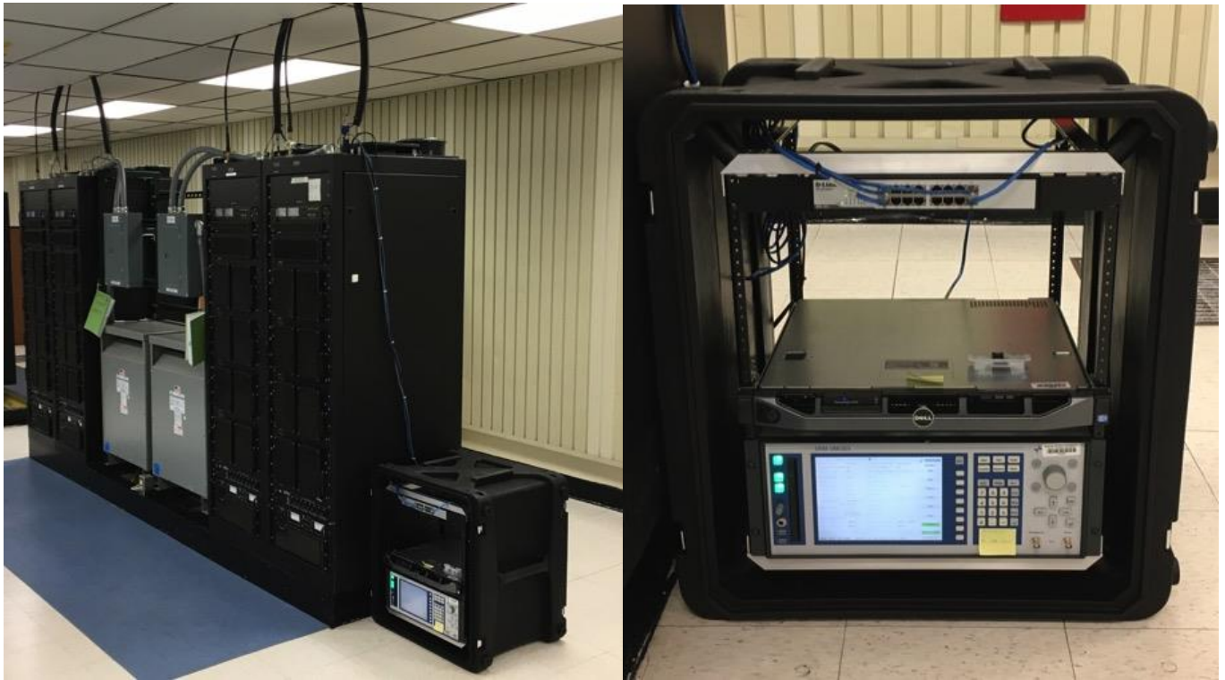
Figure 5. (Left) Kodiak HF transmitter #12 (tall cabinet on end of row closest to viewer) and portable server rack. (Right) Close-up of the portable server rack housing the content server, DMOD3 modulator, and Ethernet switch.
