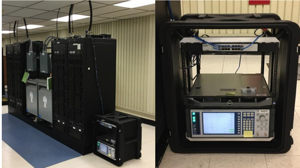
Figure B-2. (Left) Kodiak HF transmitter #12 (tall cabinet on end) and portable server rack, (Right) close up of the portable server rack housing the content server, DMOD3 modulator, and Ethernet switch.
