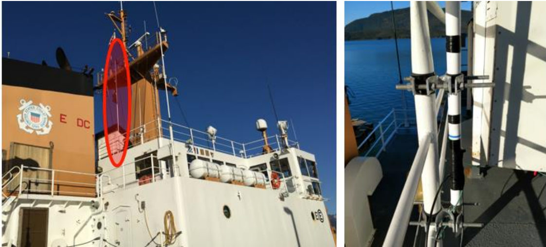
Figure B-11. Antenna (circled in red) mounted to inside of rail on deck above bridge on USCGC SYCAMORE. Close-up of rail mount on right.
