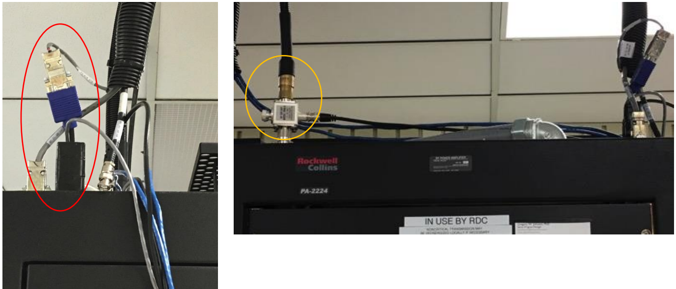
Figure B-5. Transmitter antenna interlock circled in red (left) and installed RF tap circled in orange (right).
