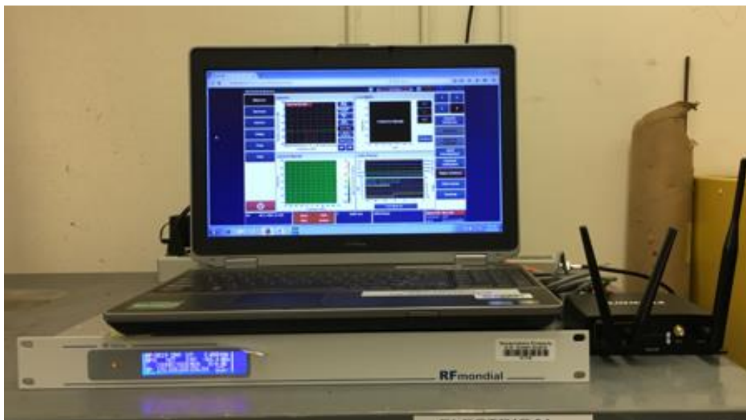
Figure 7. Alaska field test receive installation (Laptop and DRM Receiver).
