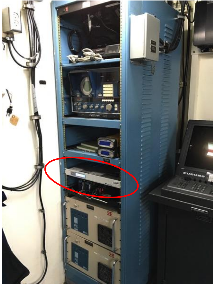
Figure B-10. USCGC SYCAMORE receiver mounted in cabinet rack in bridge chart room.
